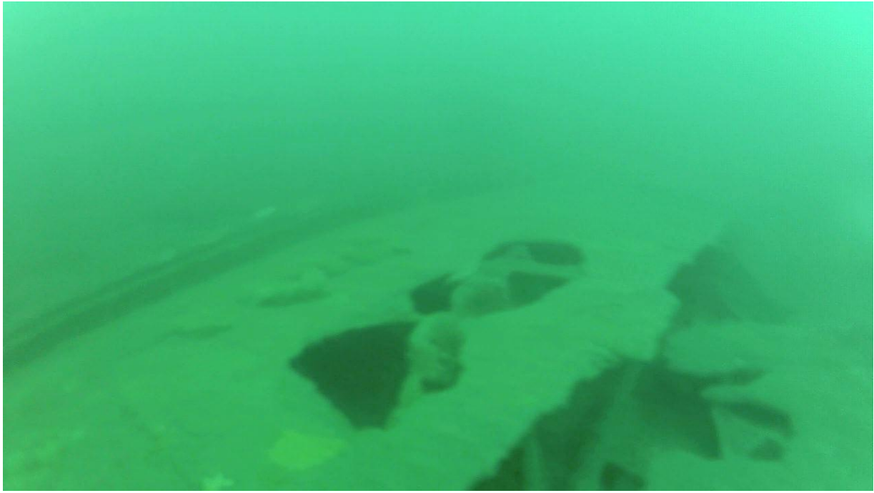
Photo 11, Hull section showing a channel appearing on the left of the photo and disappearing into the murk in the photo's centre. It probably held wooden fendering as it was located close to the deck level.
