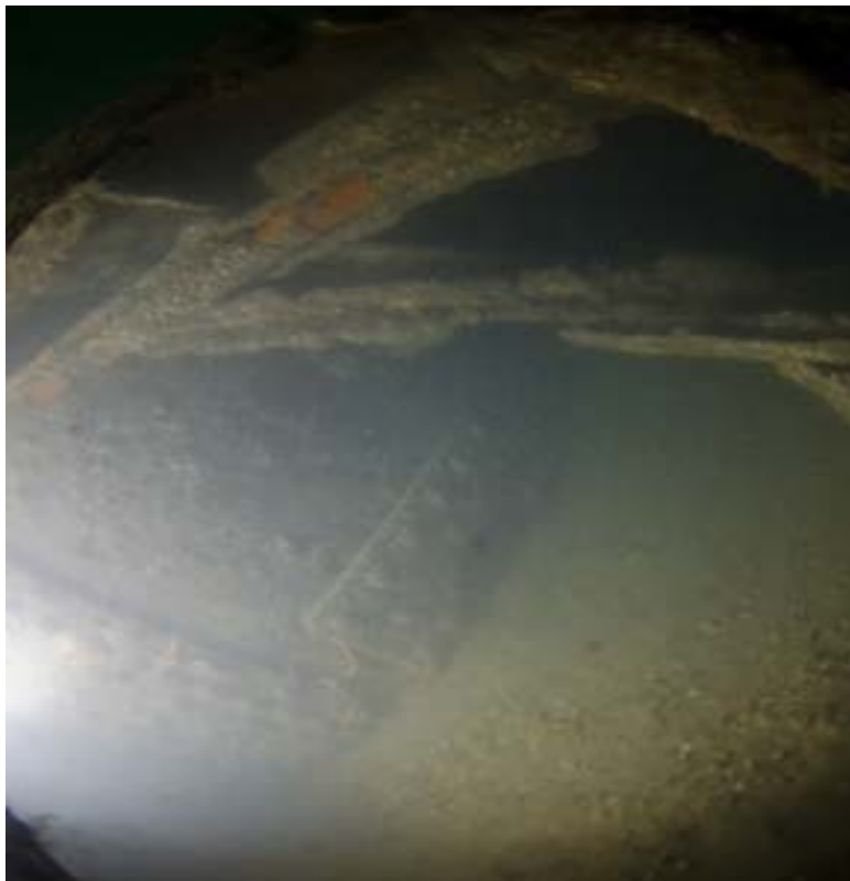
Figure 8: Looking down through broken hull plating at the port boiler
